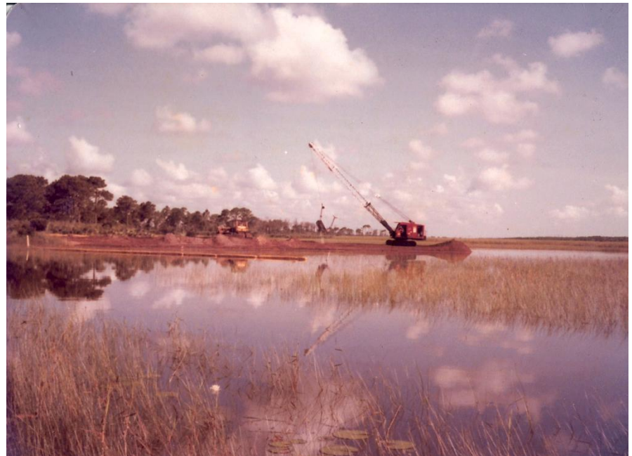
Figure 14 Working on the illegal causeway
